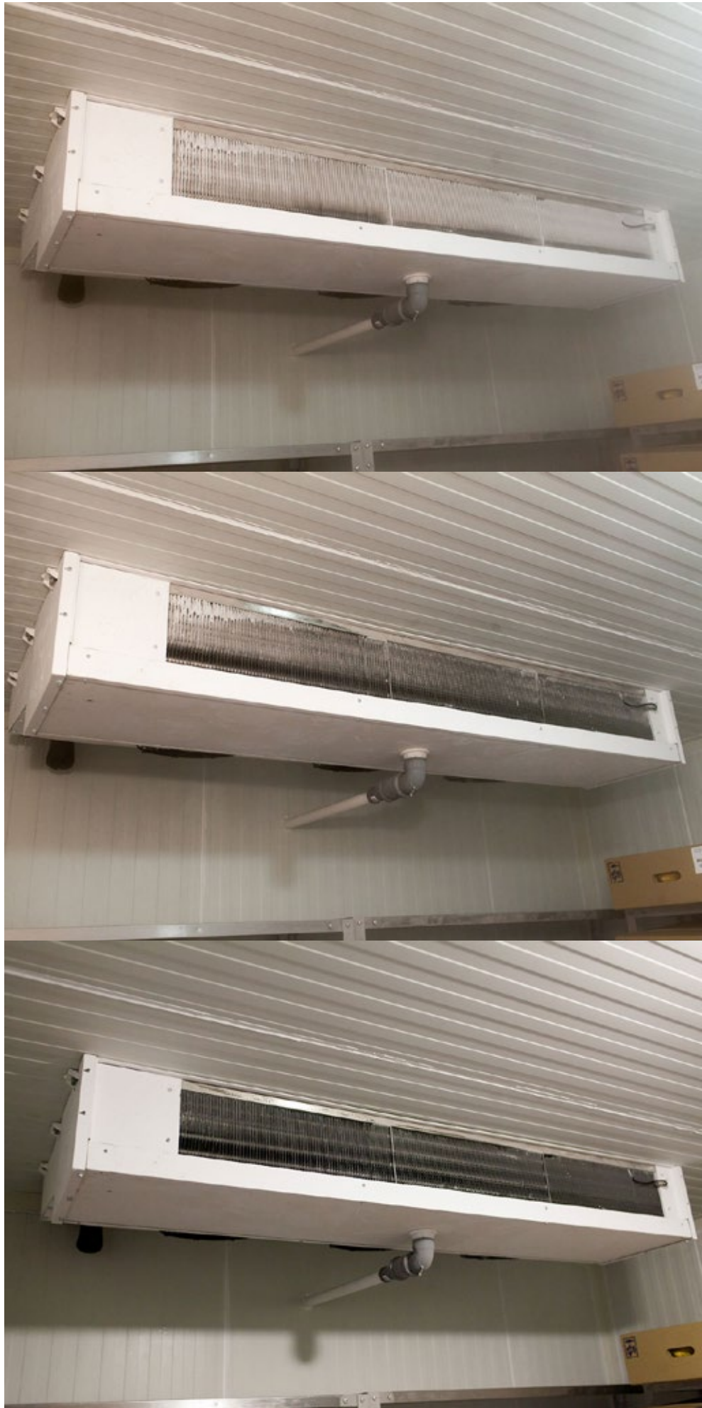
Air cooler defrosting of the low temperature chamber, which is connected to the centralized liquid defrost system and passes in 15 minutes. Brovary city, Ukraine
